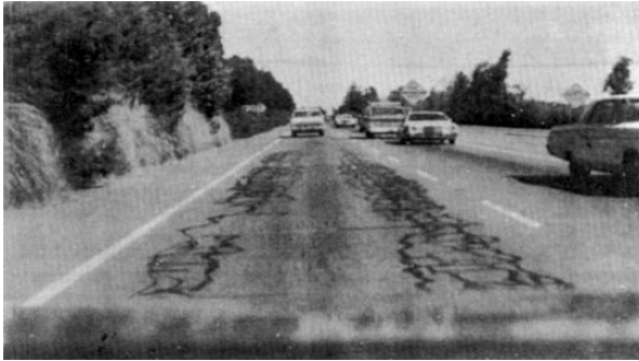
Fig. 2. Fatigue cracking in flexible pavements [6]
