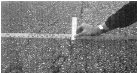
Fig. 3. Rutting in flexible pavements [6]
